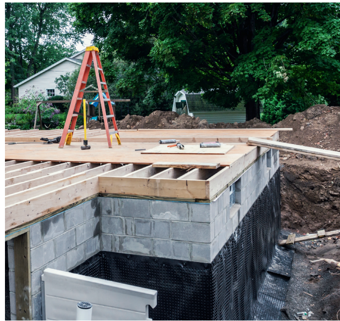
Above: This basement is being constructed in concrete-filled blockwork, with an external tanking membrane. Care must be taken during backfilling to ensure the waterproofing layer isn't punctured (by sharp aggregates, for example)
